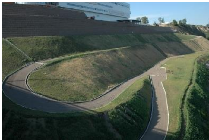
Fig. 2f. After installation and commissioning of geohazards monitoring system (Ginzburg A.A.).
